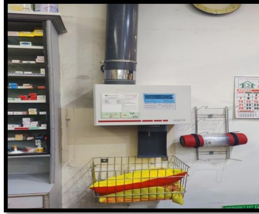
Pneumatic chute for fast delivery of medications
